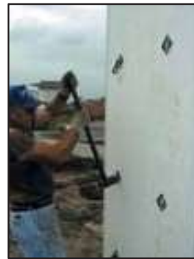
Following the order of the process, after the aluminum panel stripping, the spacers are broken with the WTF Tie Breaker Bar.
